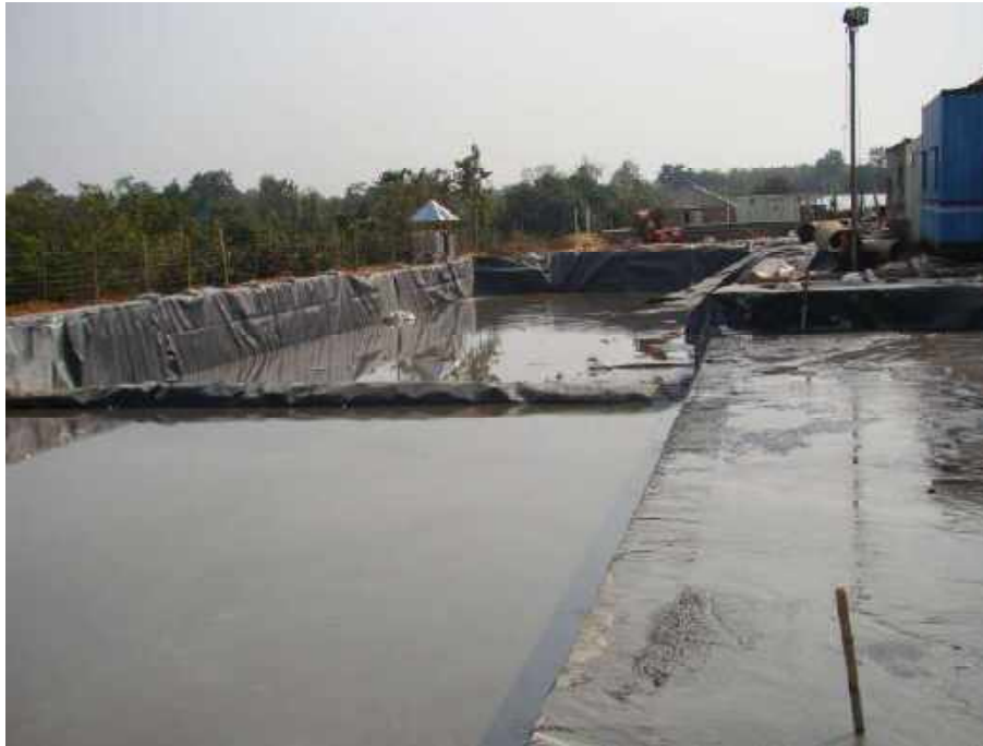
Fig. 1. HDPE lined waste disposal pits at GOAK site
