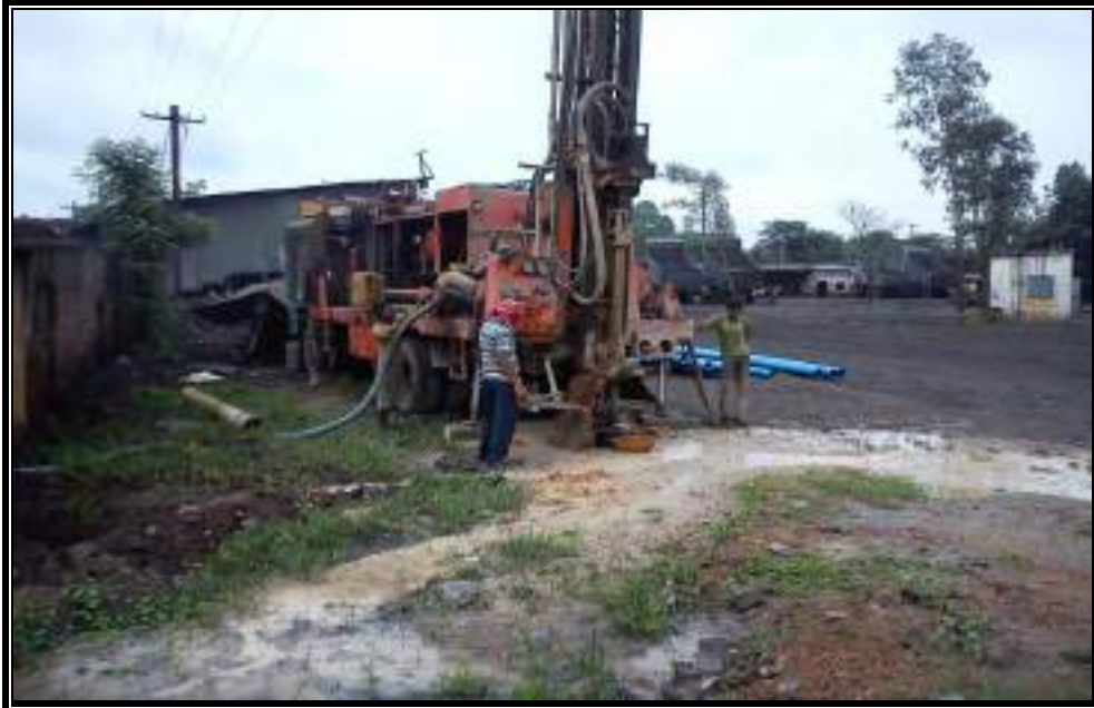
Photo 1: Exploratory Drilling Rig deployed for drilling boreholes in and around Jagannath OCP, Talcher coalfield, Odisha.
