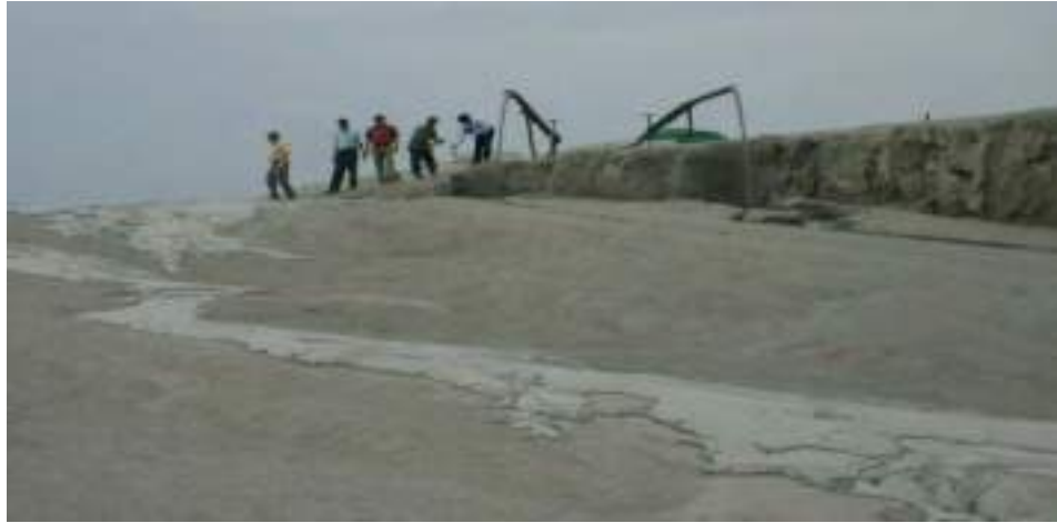
Plate 4.2: High Concentration Slurry Flowing on Slopes which dries out by the time it travels 30-40 m from the source
