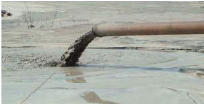
Plate 4.1: Lean Slurry Disposal System
