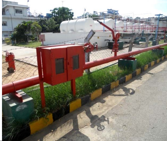
Fire Fighting system near Solvent Storage Area
