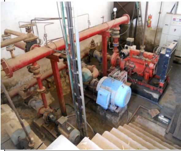
Main Pump and Jockey Pump
