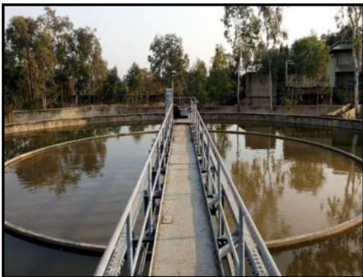
Raw water clarifier
