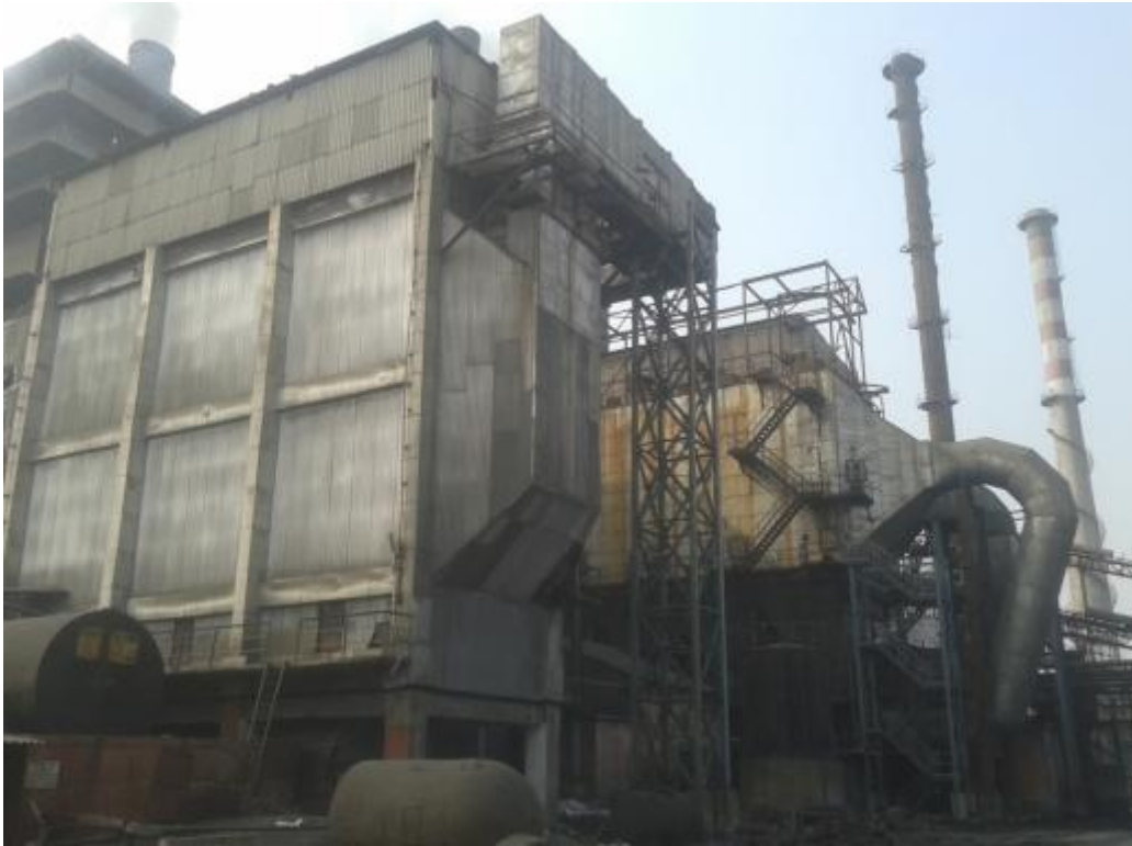
Typical View of Co-generation Boiler ESPs
