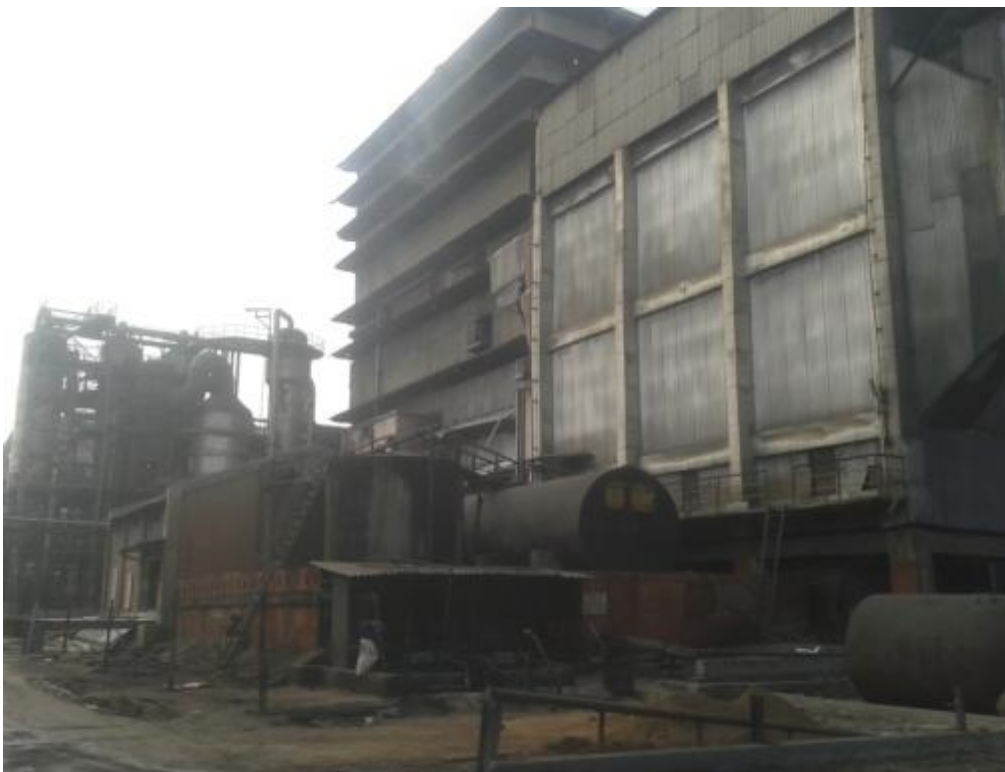
Typical View of Recovery Boiler ESP
