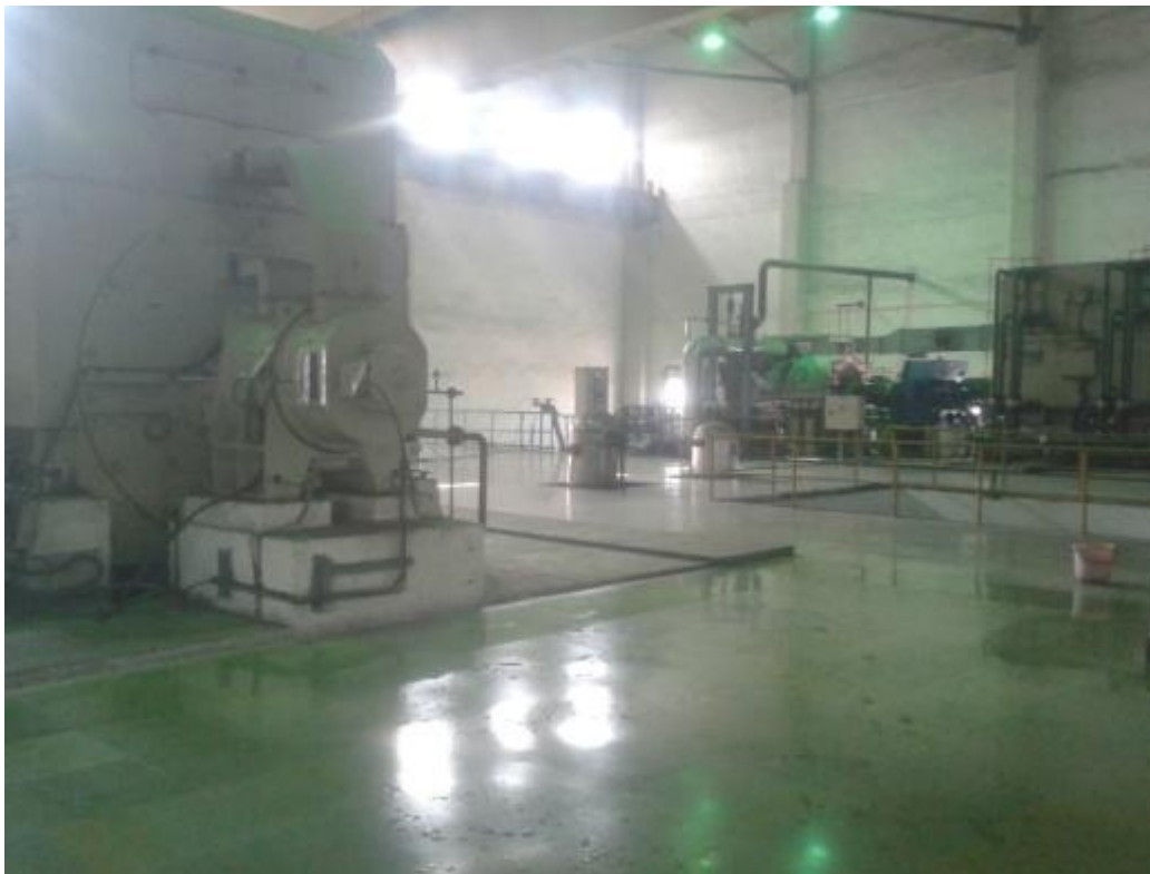
Figure 3.10 Typical View of the TG Units in the Existing Facility
