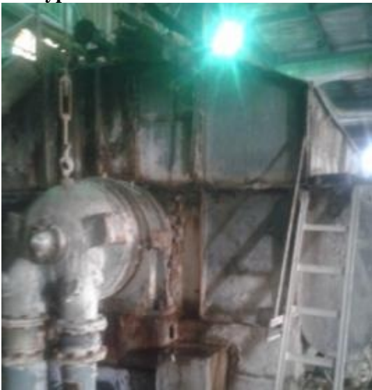
Typical View Fibre recovery and water recovery Unit in Main Paper Machine
