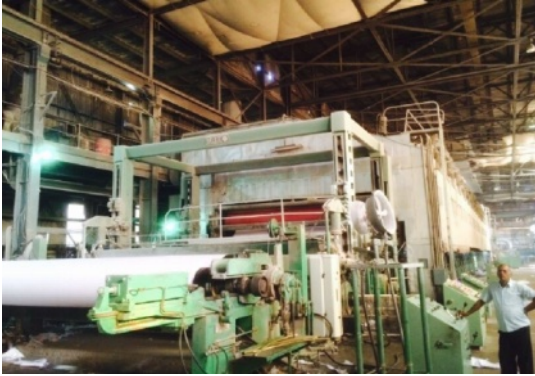
Typical View of Main Paper Machine
