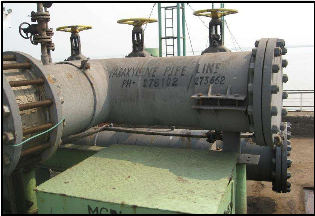
PARAXYLENE PIPELINE END MANIFOLD
