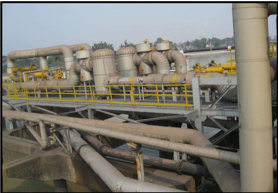
INSULATED LPG PIPELINES
