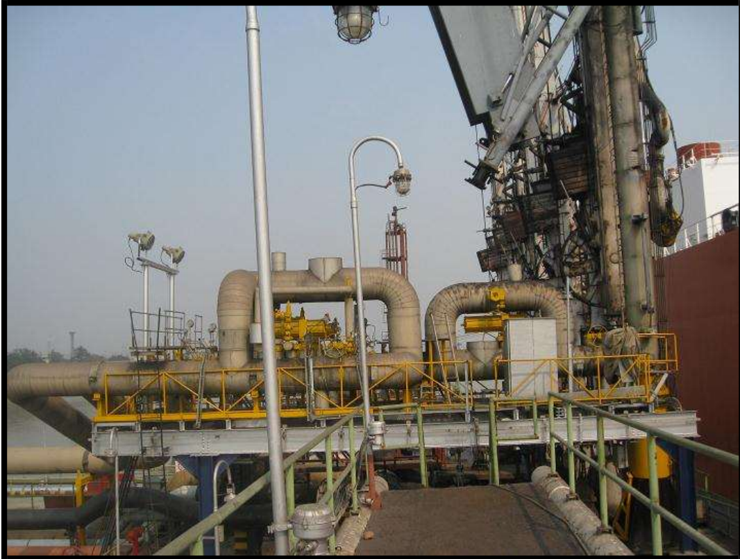
INSULATED LPG PIPELINES
