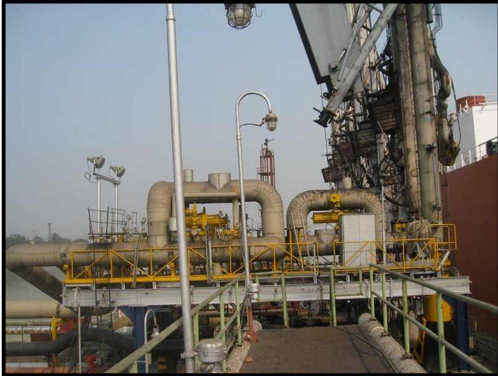
INSULATED LPG PIPELINES
