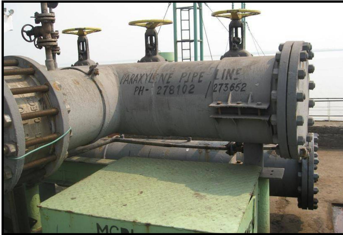
PARAXYLENE PIPELINE END MANIFOLD
