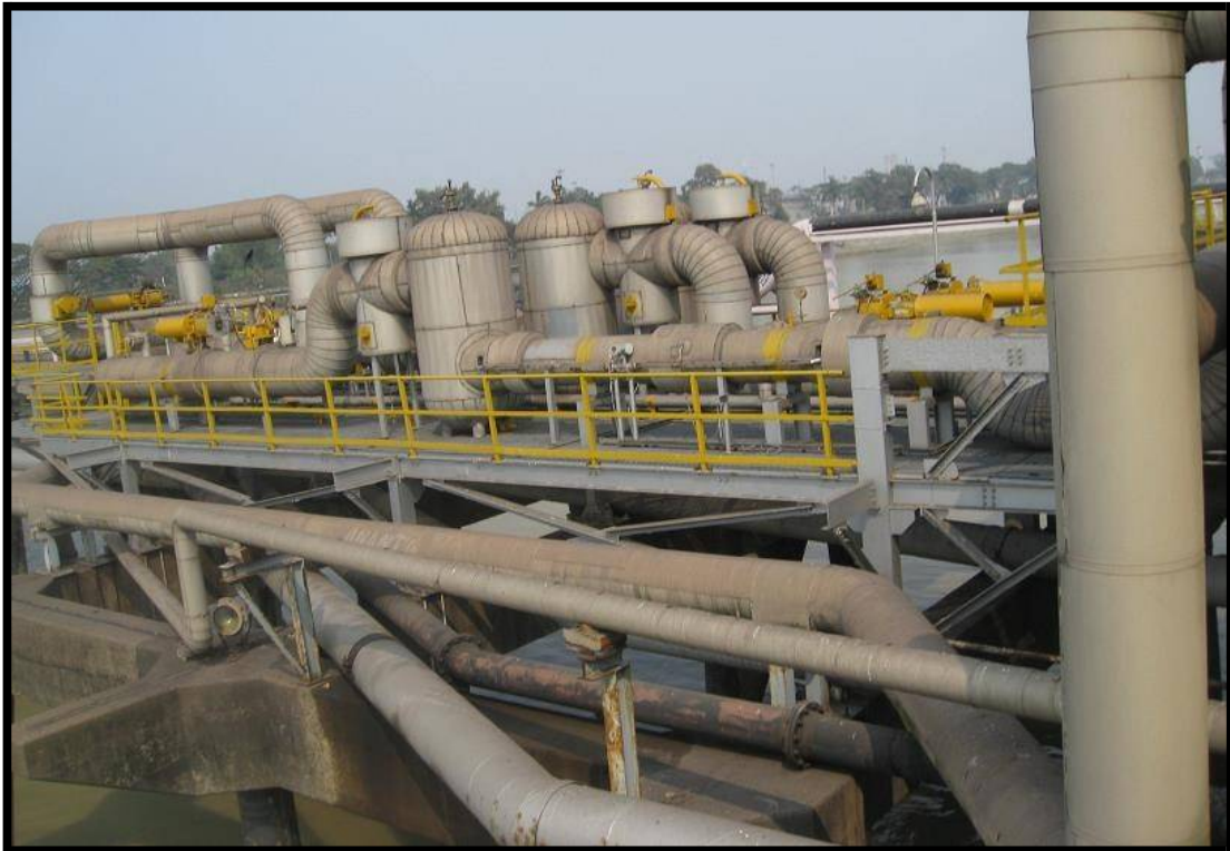
INSULATED LPG PIPELINES
