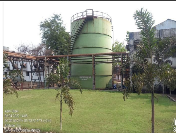
DM WATER TANK
