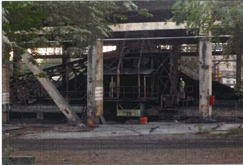
Covered Coal Storage Yard & Stacker
