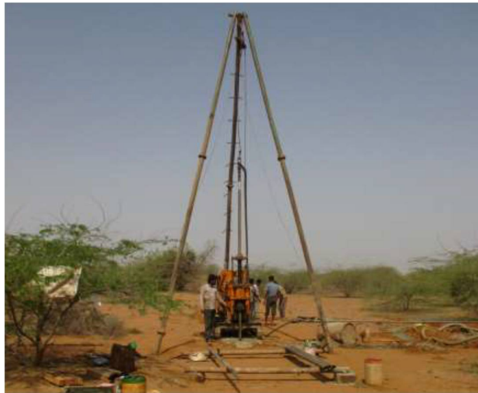
Figure:7: Voltas make, tripod mounted Drill Rigs have been used for Mudhvay Exploration
