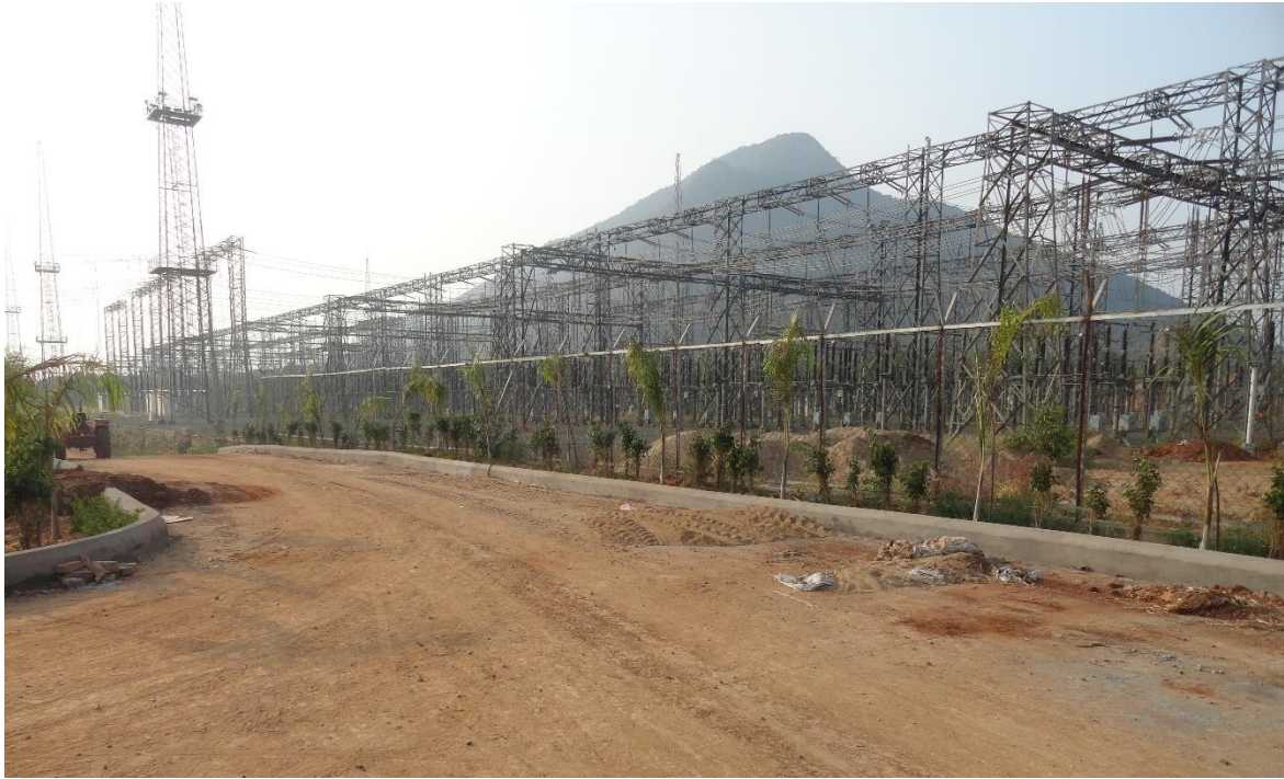
220 / 400 kV Maradam Sub-station
