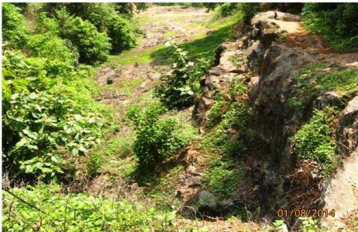
Partially completed blasting at Right flank of dam View from right flank end of dam
