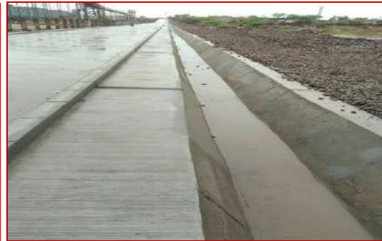
Storm water drains
