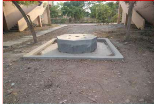
Ground Water Recharge Well
