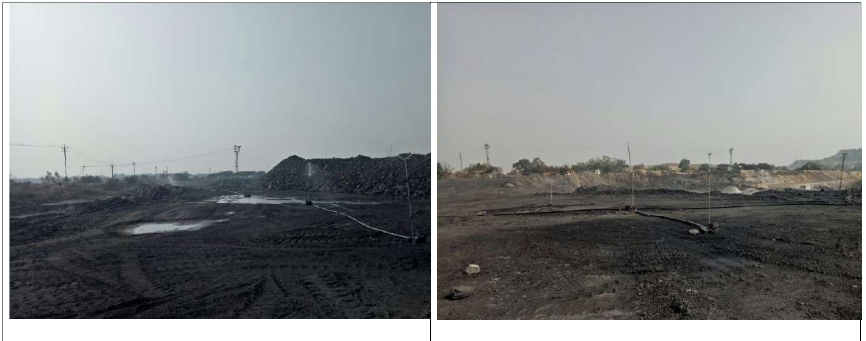
Figure 6 Fixed sprinkler at coal stock yard
