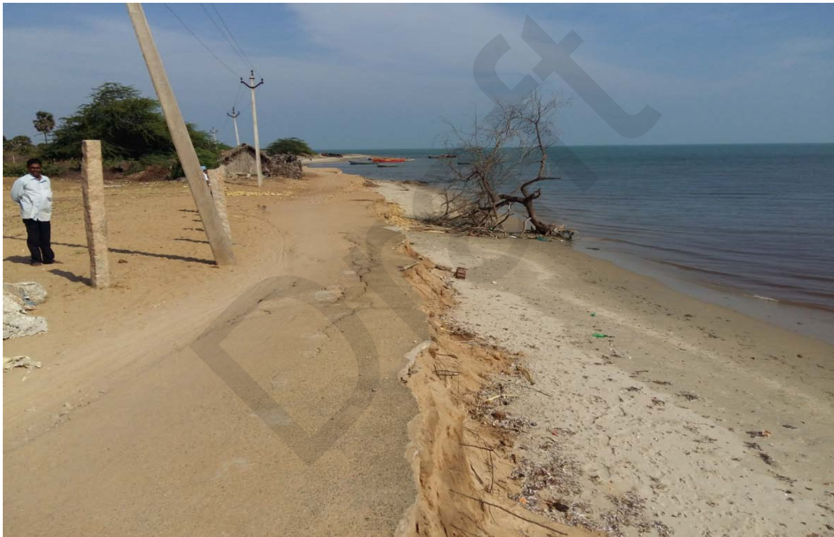
Fig.10.18a Damage of coastal road along SeeniappaDharga in Rameswaram
