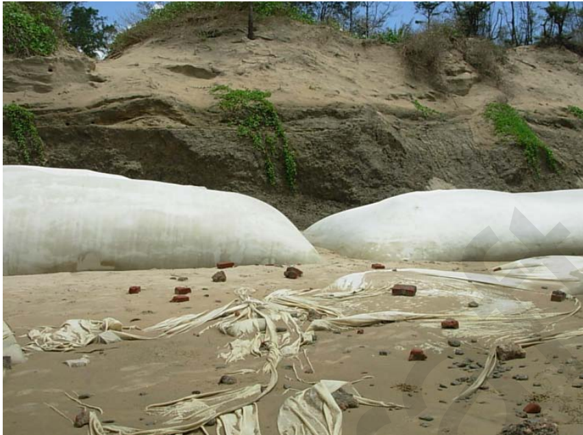
Fig.1.35a Gaps between geo-tubes- vulnerable for scour/erosion
