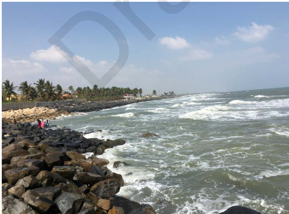
Fig.10.13e View of the existing seawall on the north of the Masilanathar temple in Tharangambadi
