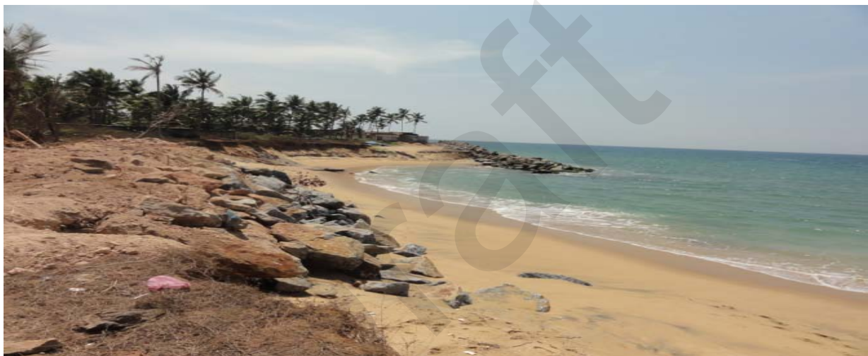
Fig.10.26 Severe erosion at Eraviputhamthurai coastal stretch
