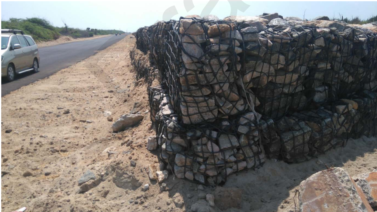
Fig.10.19b. Gabions adopted for protecting the road.
