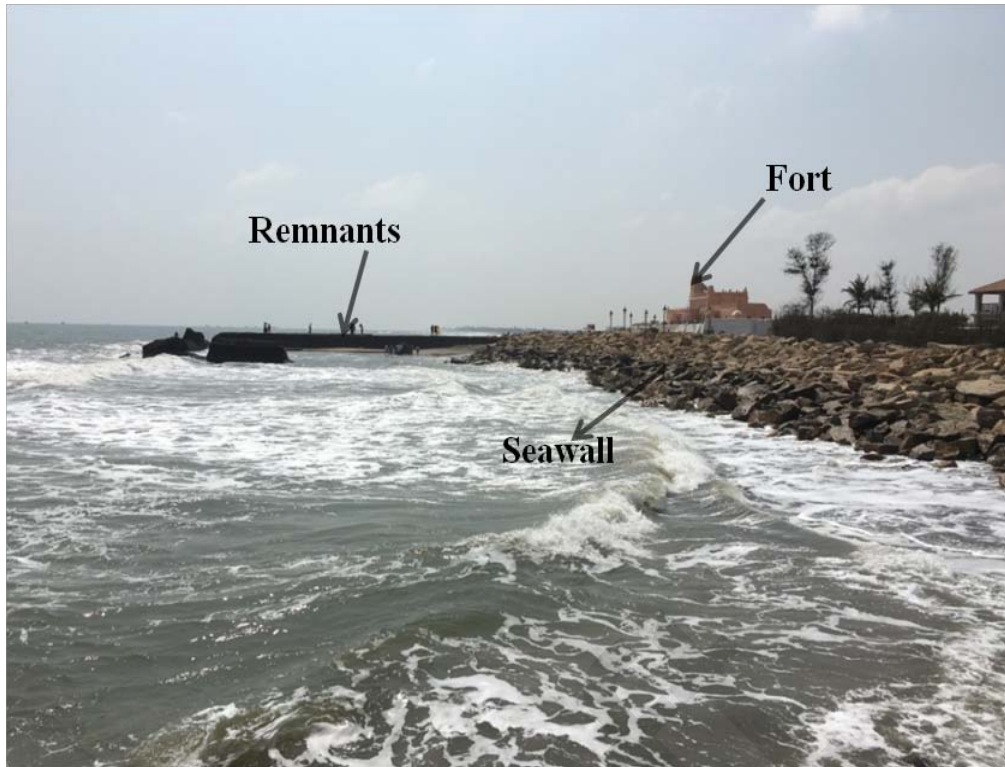
Fig.10.13d View of the existing seawall and the remnants of the building on the south of the Masilanathar temple in Tharangambadi
