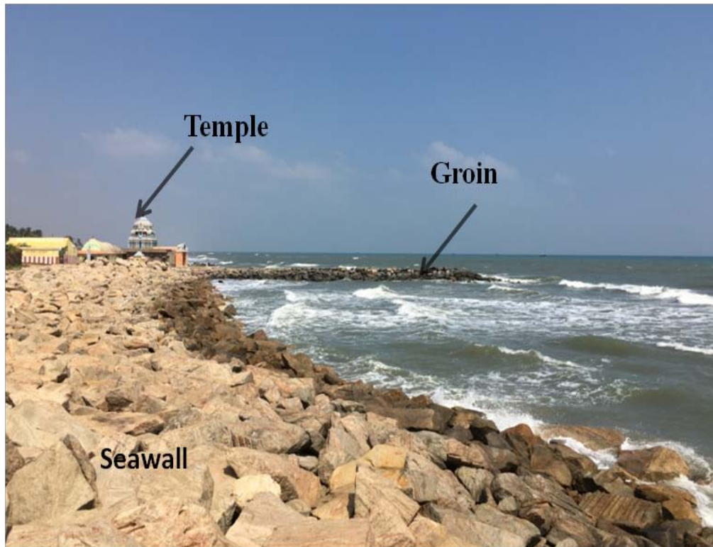
Fig.10.13b View of the existing groin in front of the Masilanathar temple in Tharangambadi
