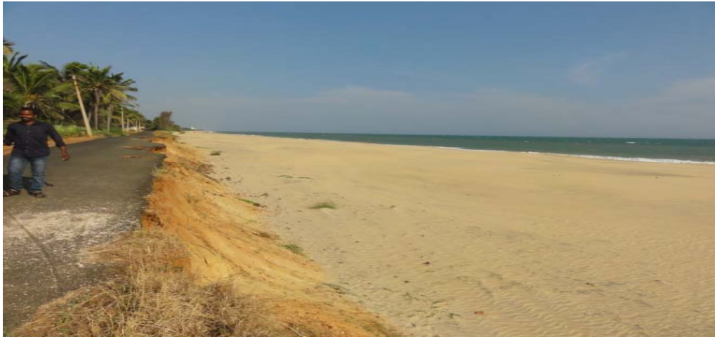
Fig.10.31a Erosion of road in Chothuvalai Beach
