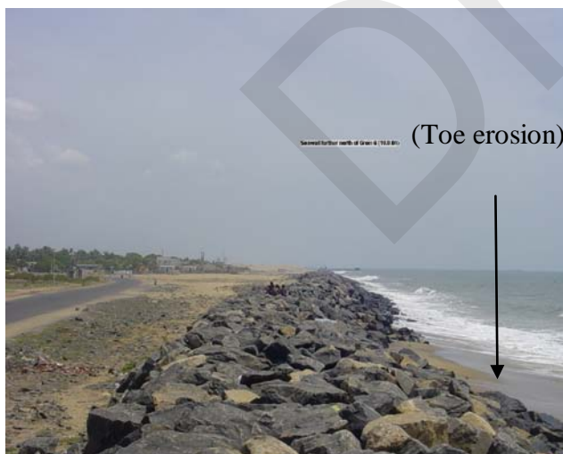
Fig.1.34. Seawall beyond ernavur experiencing toe erosion
