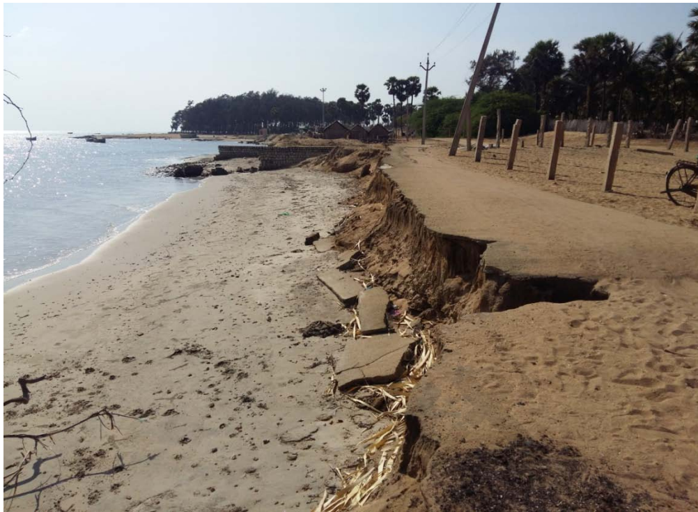
Fig.10.18b. Damage of coastal road along SeeniappaDharga in Rameswaram
