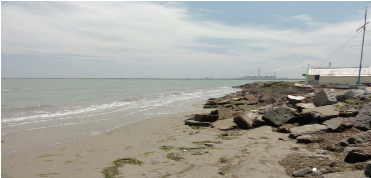
Fig.10.20b Inigonagar damaged coastal stretch
