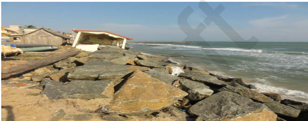
Fig.10.32b Melamanakudi coast showing the damaged seawall and the collapse of building
