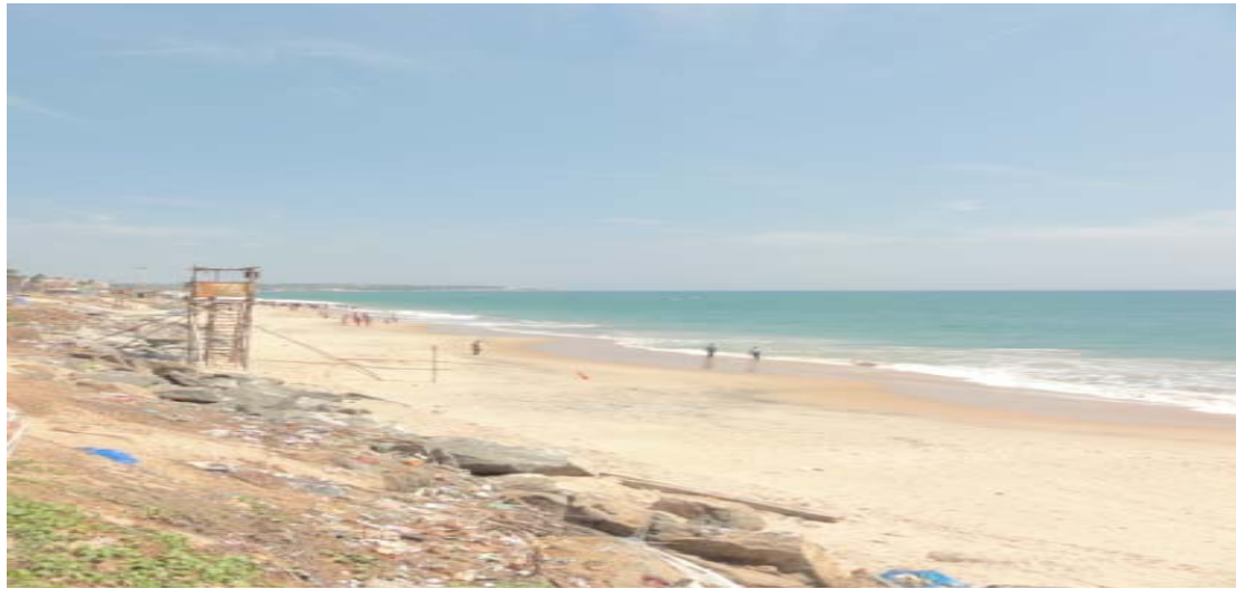
Fig.10.29b Mandaikadu Pudur coastal stretch showing the severity of the coastal berm erosion
