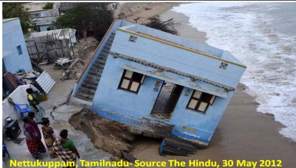
Fig.10.1c Erosion in Nettukuppam in 2012.
