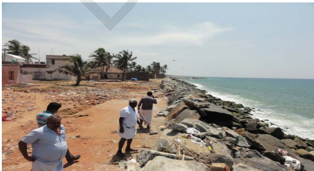
Fig.10.27c Partially functional coastal road abutting the seawall
