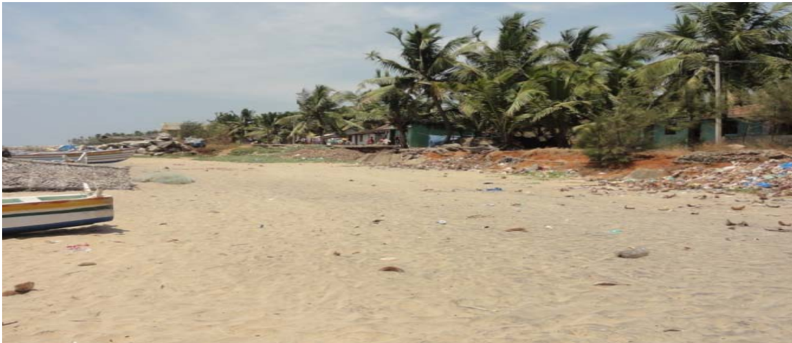
Fig.10.28a View of damaged coastal road
