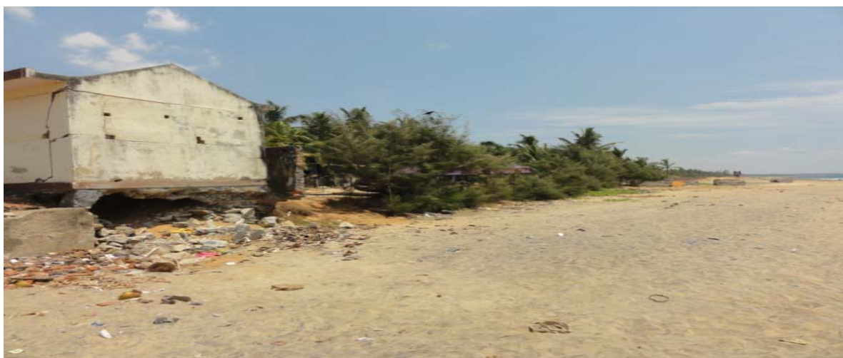
Fig.10.28c Wave scouring the building foundation
