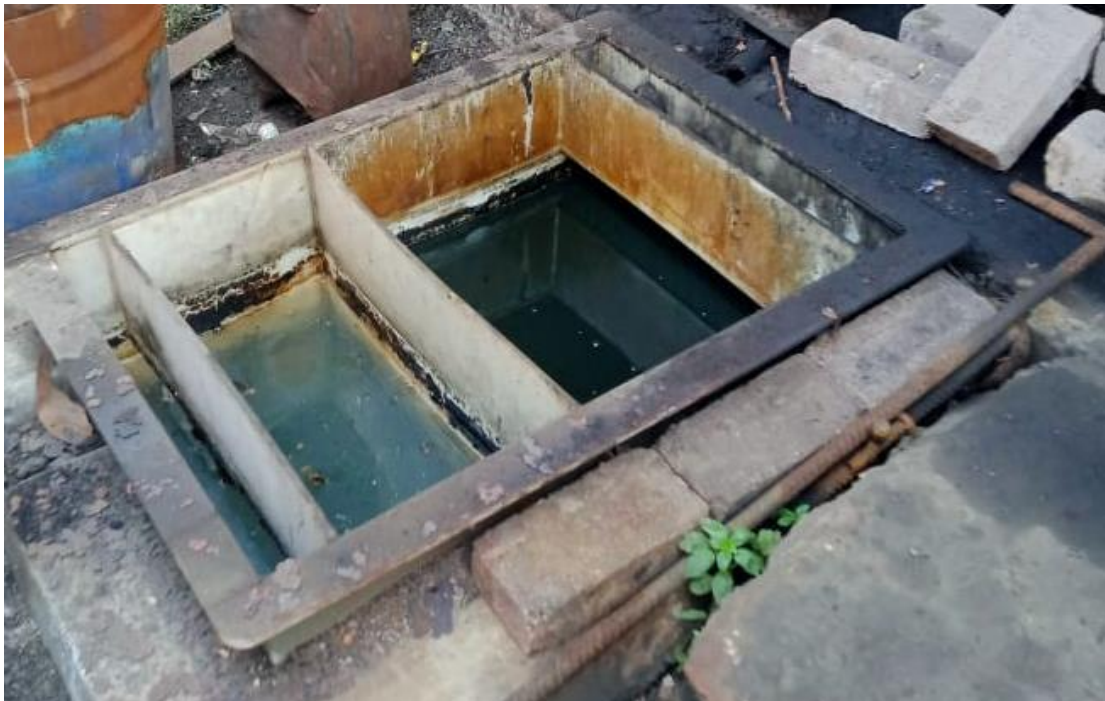
Oil and Grease Trap at Bankola Workshop
