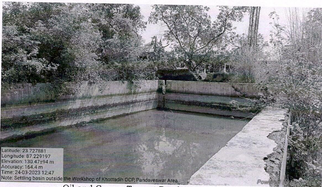
Oil and Grease Trap at Pandaveswar Workshop
