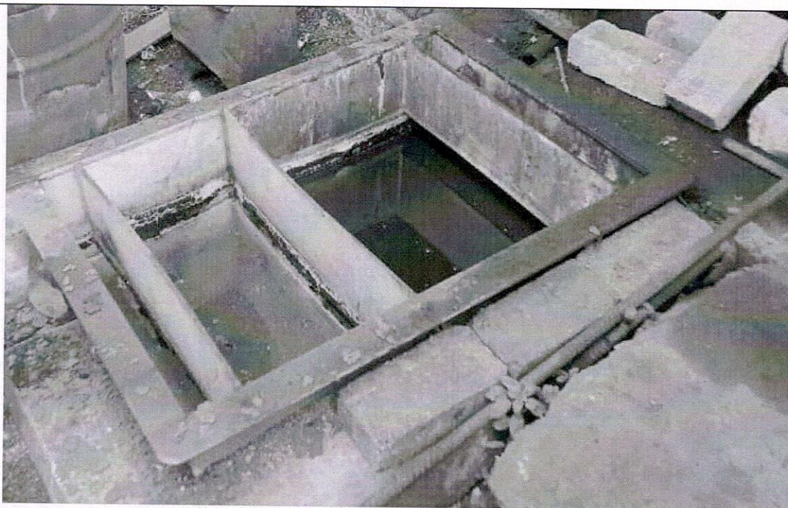
Oil and Grease Trap at Bankola Workshop
