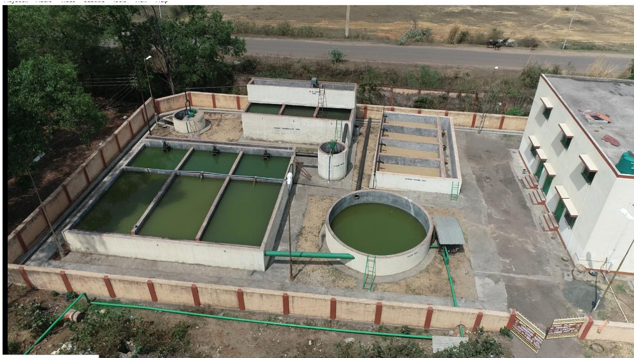
ETP at Workshop under Sonapur Bazari Area
