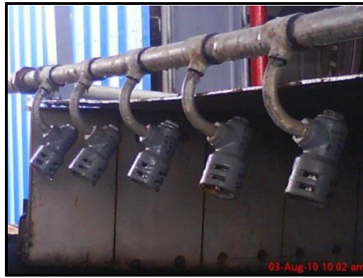
Cone Nozzles at Hopper
