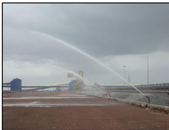
Water Sprinklers/Dust Suppression at stockyard
