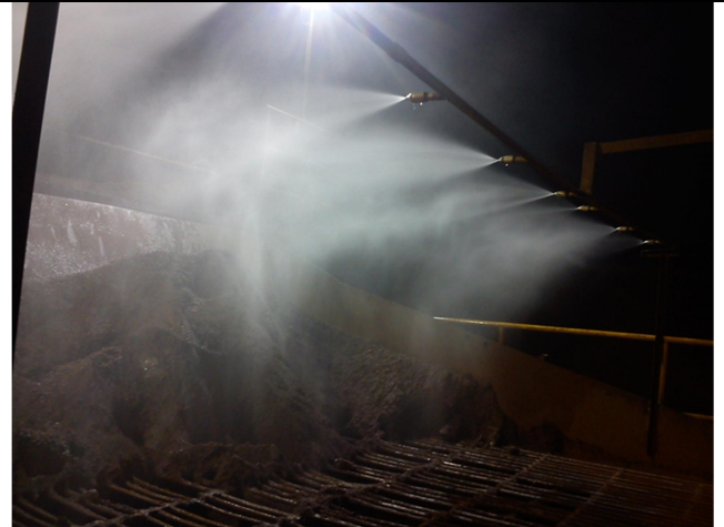
DRY FOG SYSTEM AT BENEFICIATION PLANT
