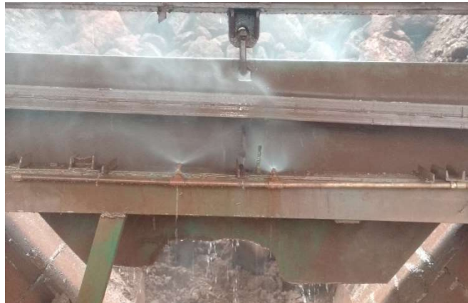
DRY FOG SYSTEM AT CRUSHING PLANT
