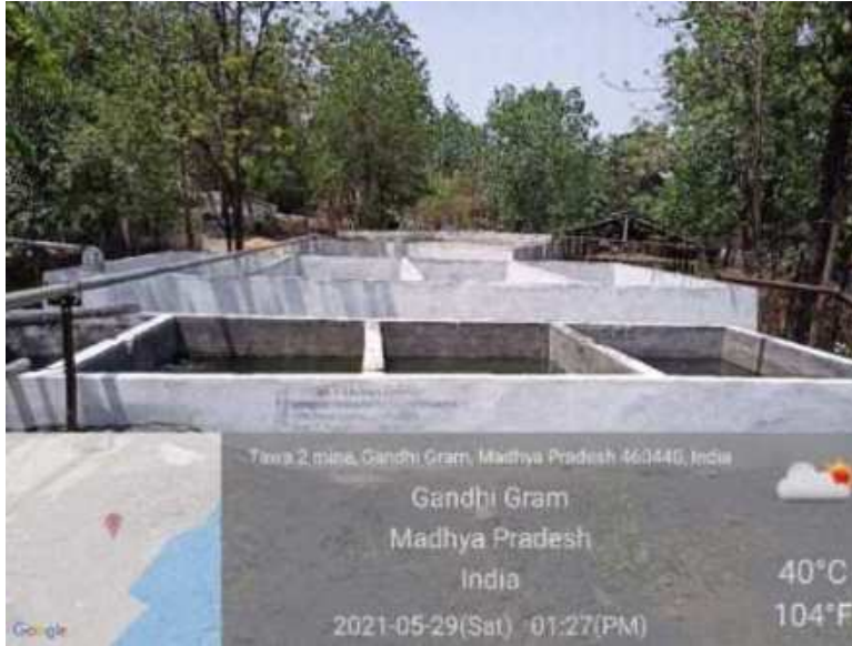
Figure 3 Sedimentation tanks at Tawa-II UG mine
