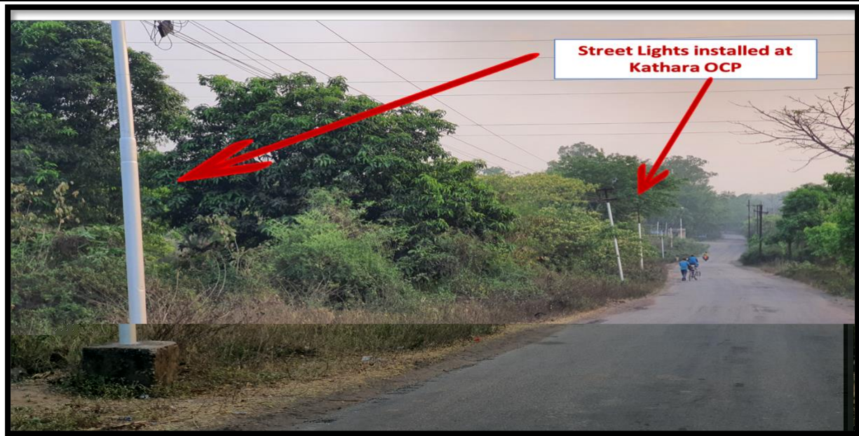
60-watt LED street light installed near Kathara OCP
