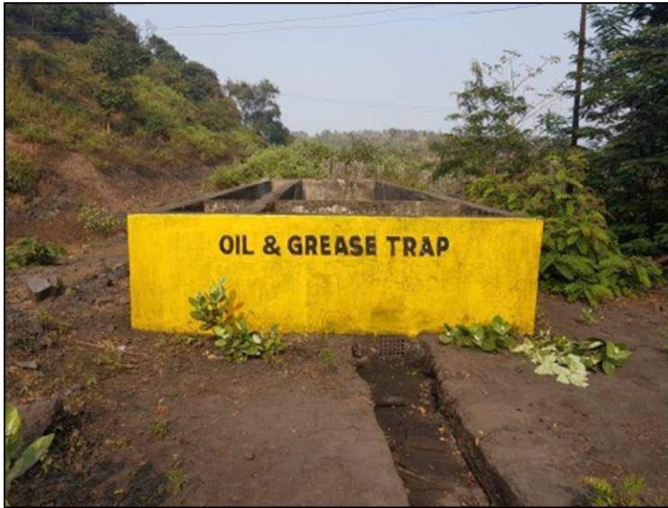
Fig: Oil and Grease Trap at Karo OCP
