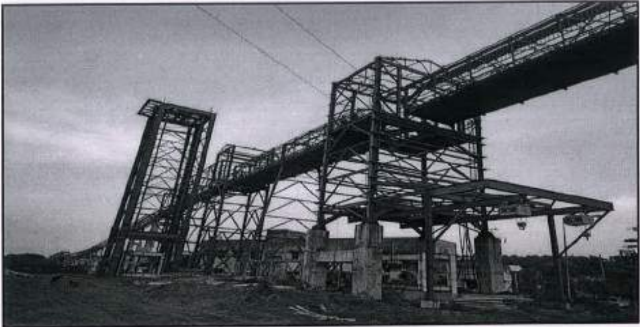
Coal Pipe Conveyor System
