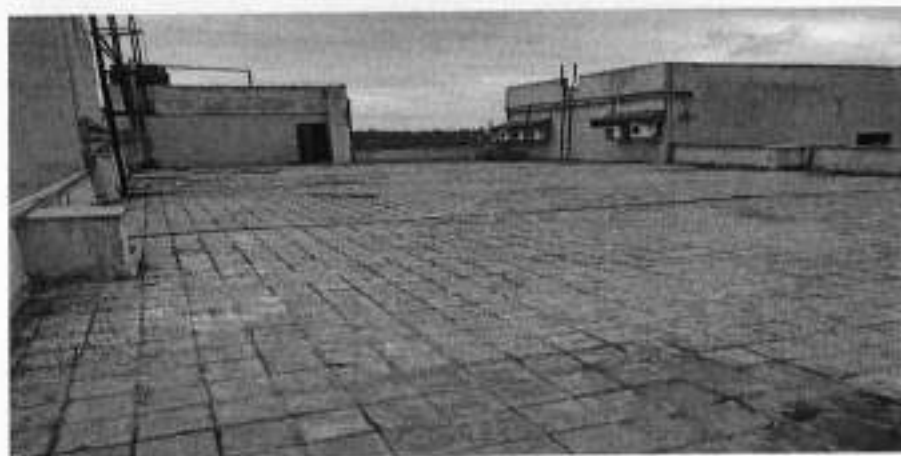
13. CW Pump House Terrace
