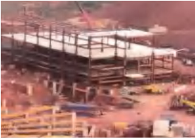
Pump House ECR
