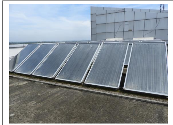
Solar Water Heating
