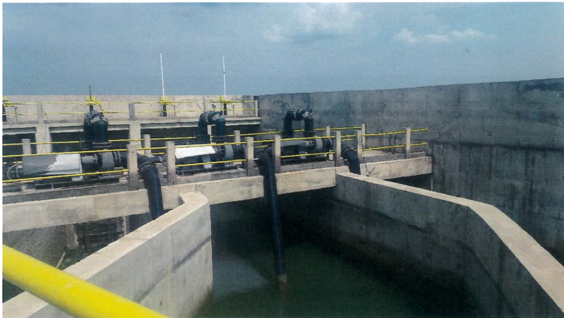
Figure 2. Seawater intake structure (common to both phases)
