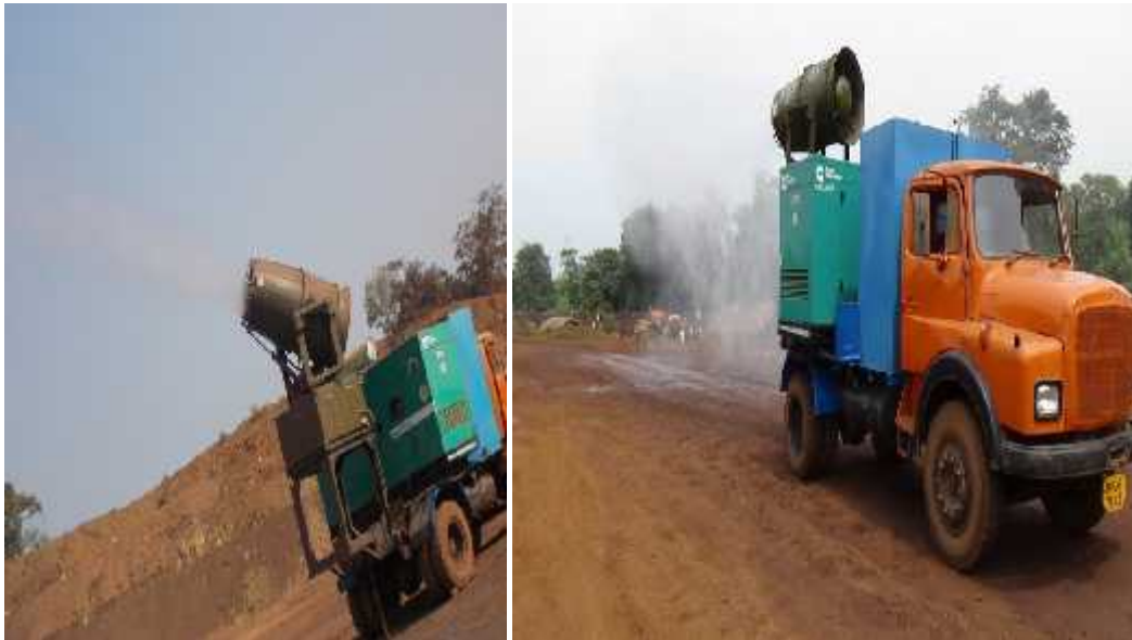
VIEW OF WATER TANKER AND FOG MACHINE BEING USED FOR WATER SPRINKLING PURPOSE
