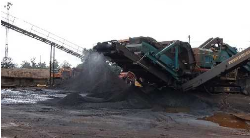
MOBILE CRUSHER PLANT WITH WATER SPRINKLING SYSTEM
