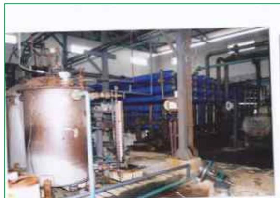
Ultra Filters at ETP-RO
