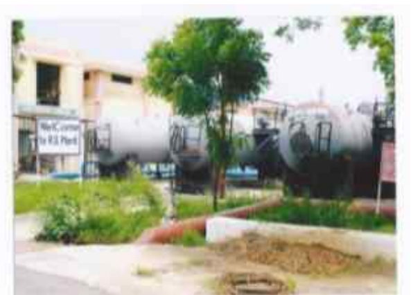
Activated Carbon Filters
