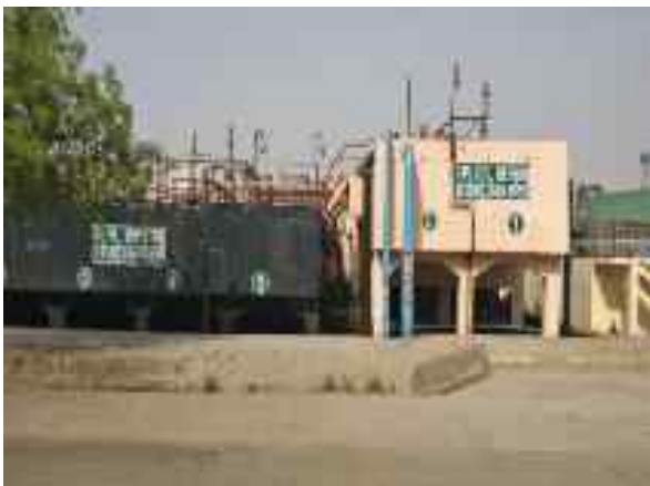
API Oil Separators
