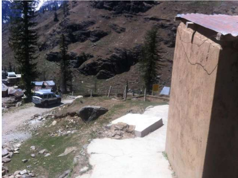
Figure 7.11: Location of proposed Lower Terminal at Kothi Flood/Land slide Hazards; near Nalla passing near LTP L
