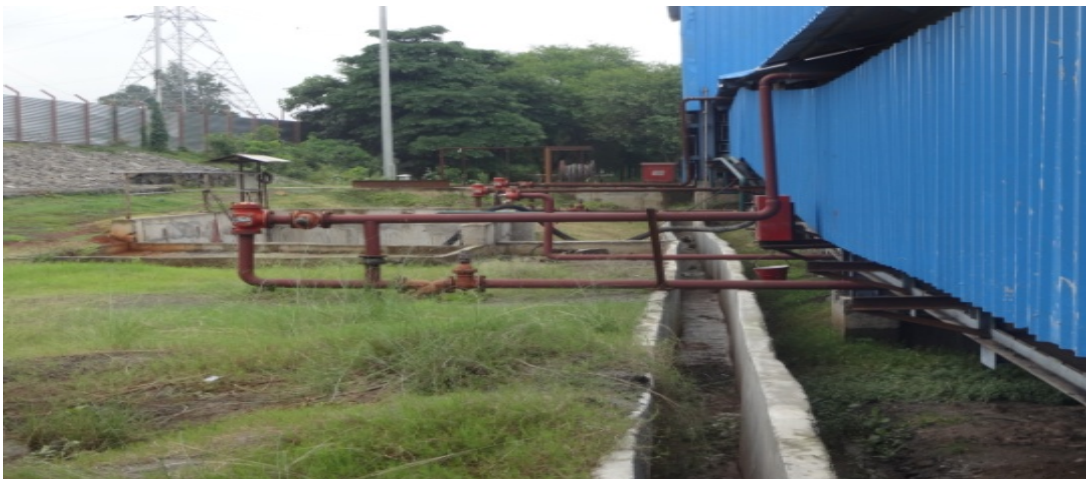
Fig. 11. Collection system for coal slurry
