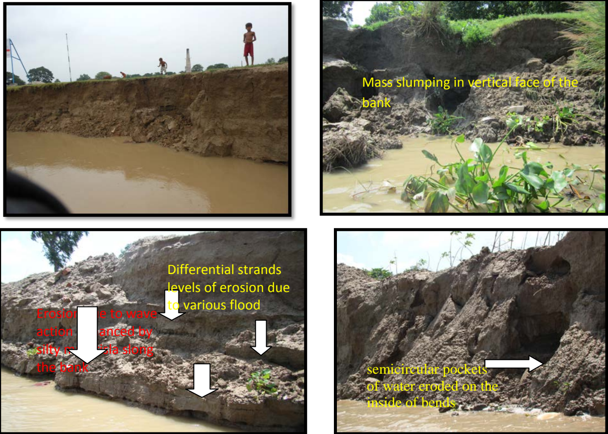
Fig. 103. A view of the vertical face of the bank eroded by mass slumping due to undercut action
