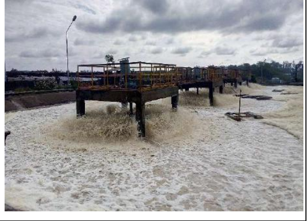
ETP- Aeration Tank
