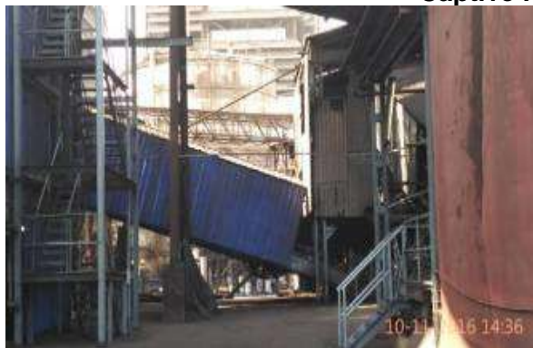
Closed Coal Conveyor
