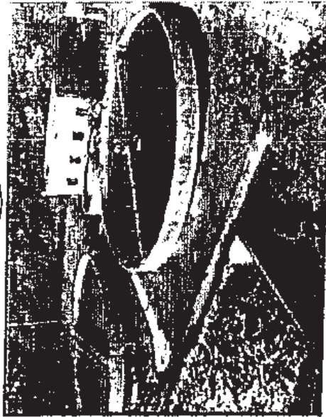
Plate 1.3 Effluent Treatment Plant Tanks
