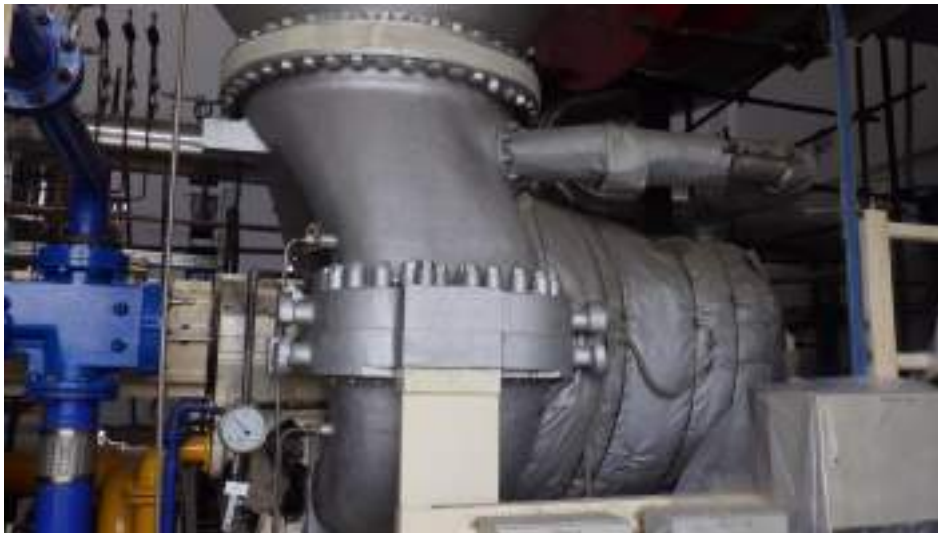
Figure No. 7.11 Turbine
