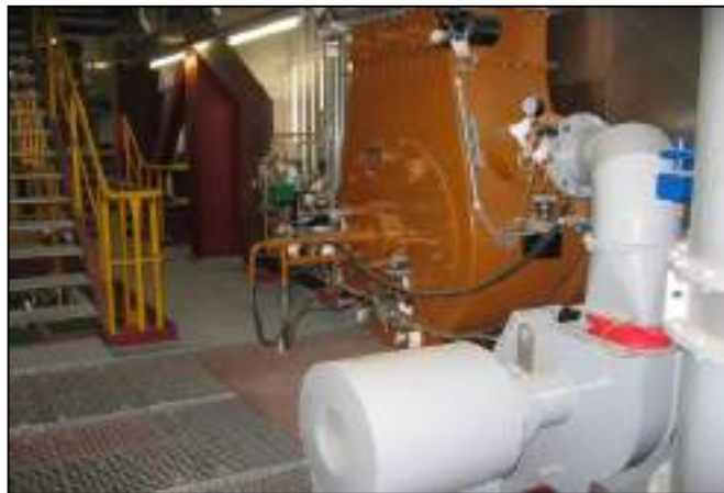
Figure No. 7.7 Startup Burner
