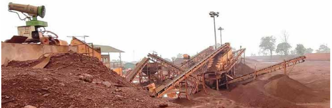
Fig.4.3: Misting Cannon (far left) at Mobile Crushing & Screening Plant, Kalta Mine
