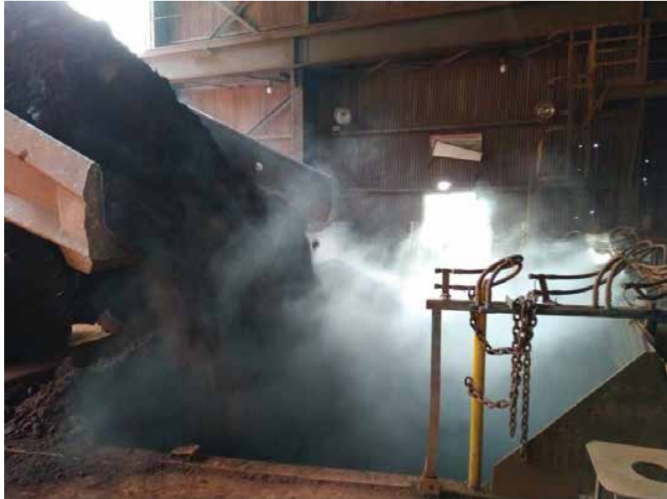
Fig.4.2: Dry Fog Dust Suppression System at Receiving Hopper, Barsua Beneficiation Plant
