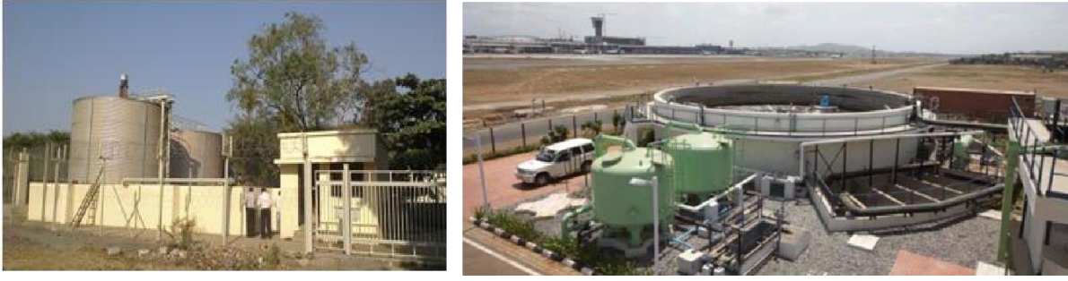
Figure 2-7: Photographs of constructed STPs on site as part of the sewerage layout of landside development
