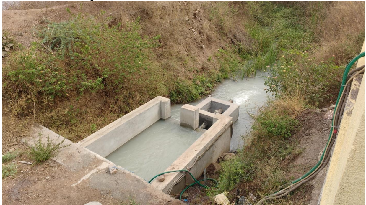
4. Ashwater discharge and online monitoring point
