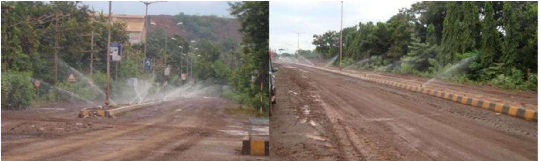
Stationary Water Sprinkler
